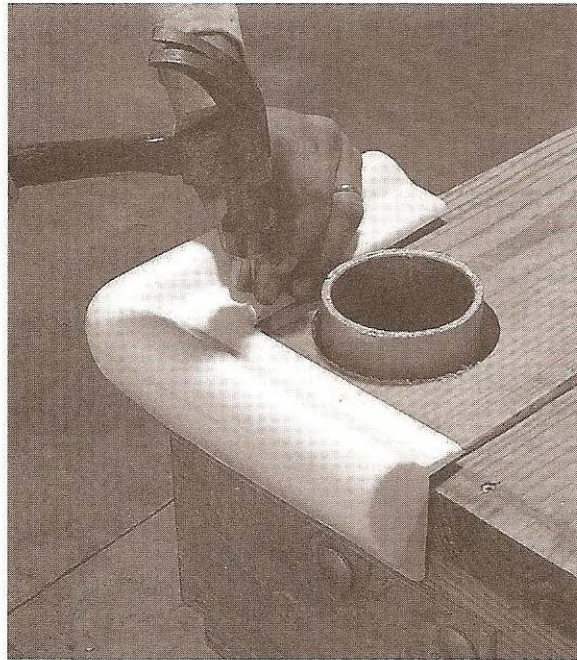
30. Nail down outside corner bumpers with stainless ring shank large head nails. Four nails on top and four nails on the bottom.
