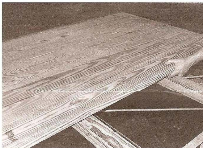
24. Lay down deckboards tight together. If you are using 2" x 6" that are wet, they shrink about 1/4" and leave a nice drainage crack.
