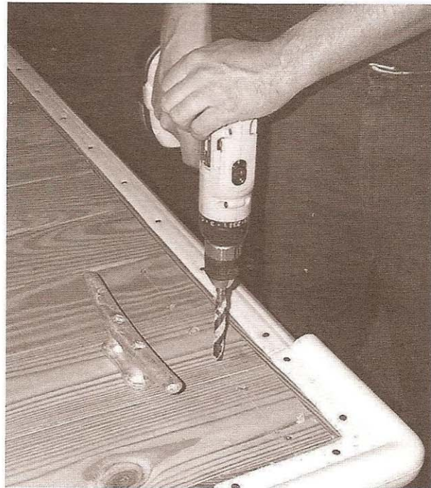
29. Drill and attach cleats. Drill cleats next to truss frame, but not through angle. Use large washer that will clamp over 1/2 of the angle. See below.
